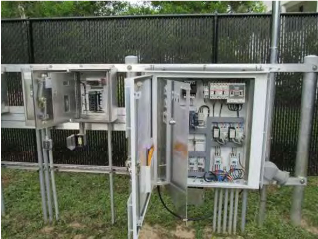
Figure 3-4. Photograph of Lift Station Control Panel Interior.
