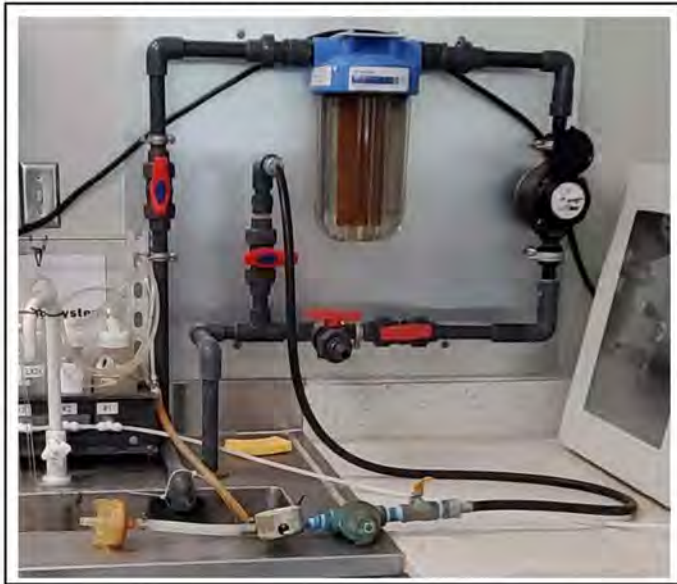
BFI Device in MAR Facility Lab
