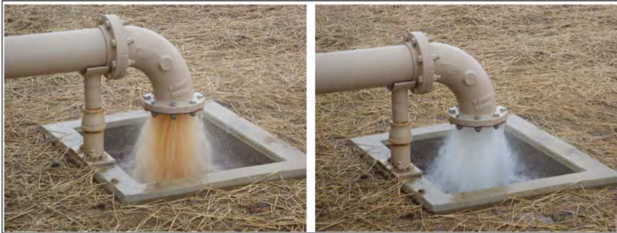
Figure C-9. Example of Backflushing Discharge.
