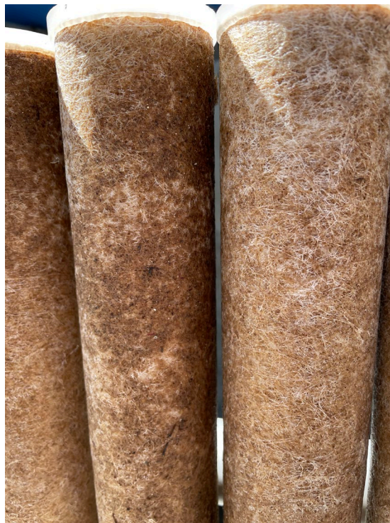
Figure 5-7. Cartridge Filters After Changeout on February 24, 2021.
