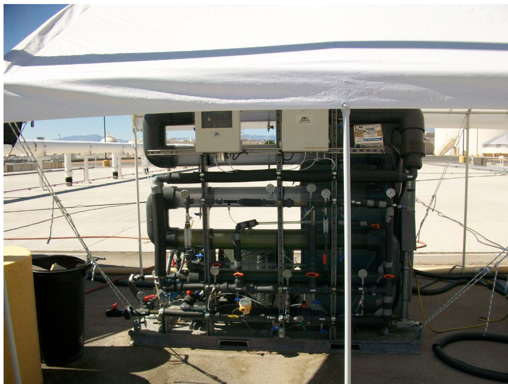
Figure 4-5. An Example Pilot-scale Ozone System with Built-in Serpentine Pipeline Contactor.
