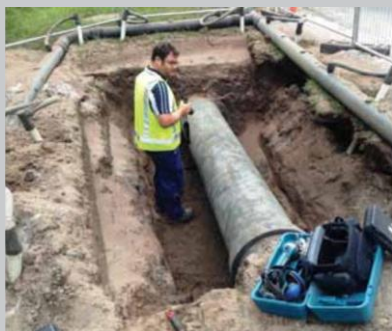
Figure 1. Collecting soil and other data at an open pit in the Hunter Water network (Photo courtesy of Hunter Water)
