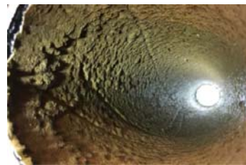
Interior of removed pipe section showing thin scale
